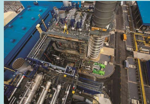
NongSang Power Plant 9,119 THBmn, Gulf Electric
