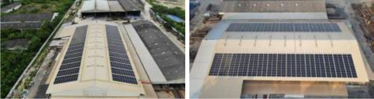
Photo depicting an applying Solar rooftop in our area.
