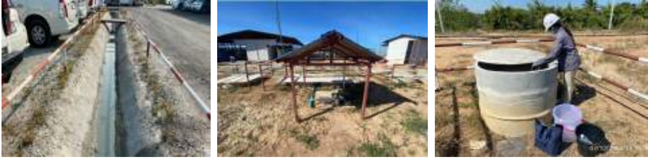
Photo depicting temporary water drainage ditches, temporary wastewater treatment system, and monitoring of wastewater quality in the project site
