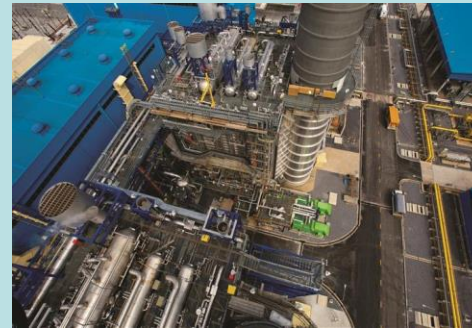
NongSang Power Plant 9,119 THBmn, Gulf Electric
