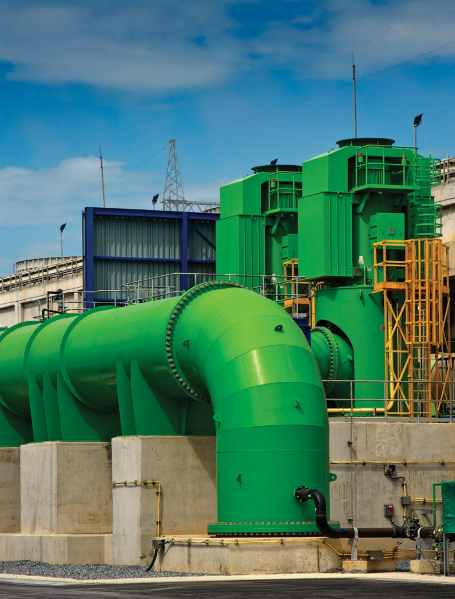
Nong Saeng Power Plant, Saraburi
