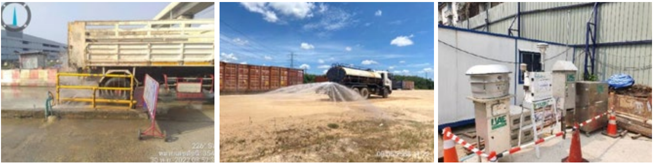
Cleaning wheels before leaving the construction area, spraying water to reduce dust diffusion, and measuring the air quality within the construction project area.
