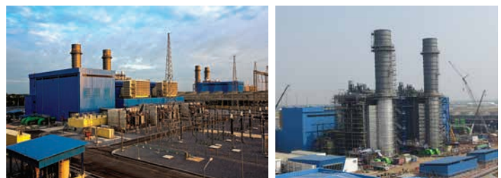
GJP-GNS and GUT combined Cycle Power Plants
