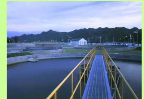
Waste Water Collection & Treatment Plant 740 THBmn, Municipal of Nakorn Ratchasima
