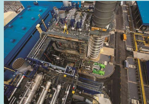
NongSang Power Plant 9,119 THBmn, Gulf Electric
