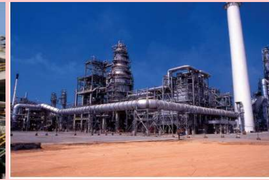
Thaioil Hydrocracker (HCU)-2 538 THBmn, Chiyoda
