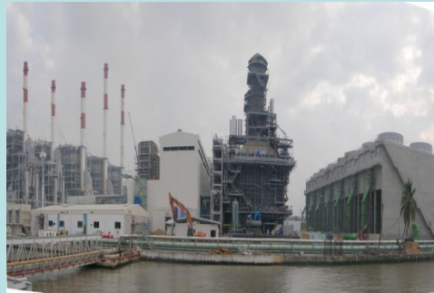
South Bangkok Power Plant 2,300 THBmn, EGAT
